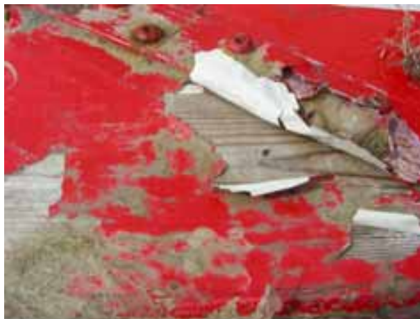
Peeling paint on the wooden float
