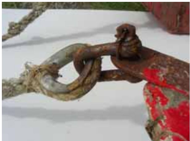
Paint damage on the mooring bridle
