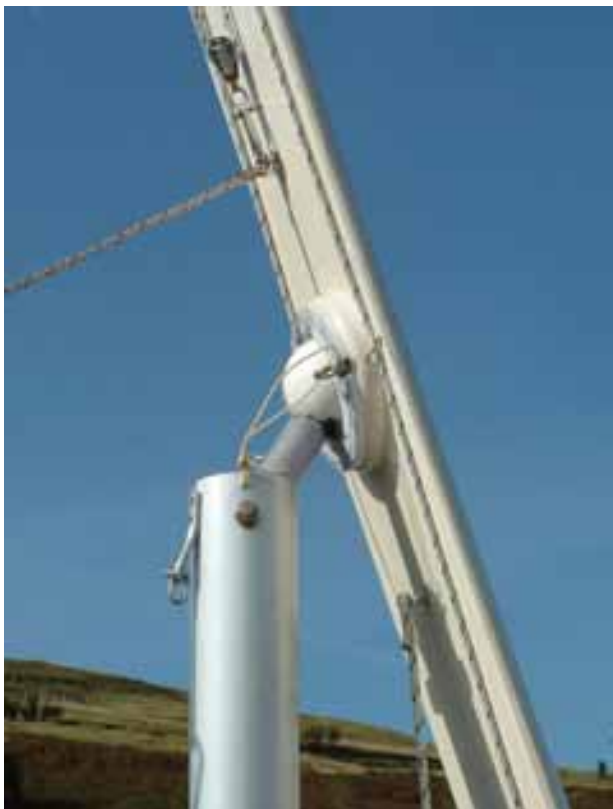
Photo 1 - mast top ball and socket joint
