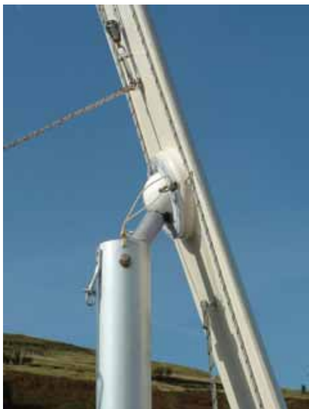
Photo 1 - mast top ball and socket joint
